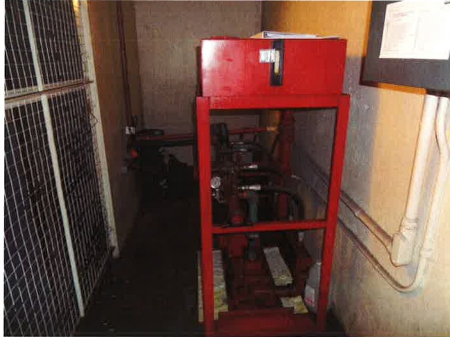
Photograph 5: View of the hydraulic cage for the elevator. Minor staining which is absorbed via sorbent cloth. Equipment appears to be well maintained
