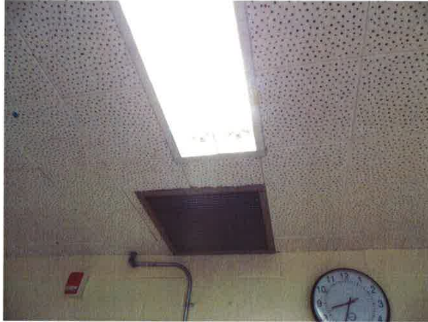
Photograph 11: Fluorescent lights and return air. Lay-in ceiling tiles were observed in the classroom.
