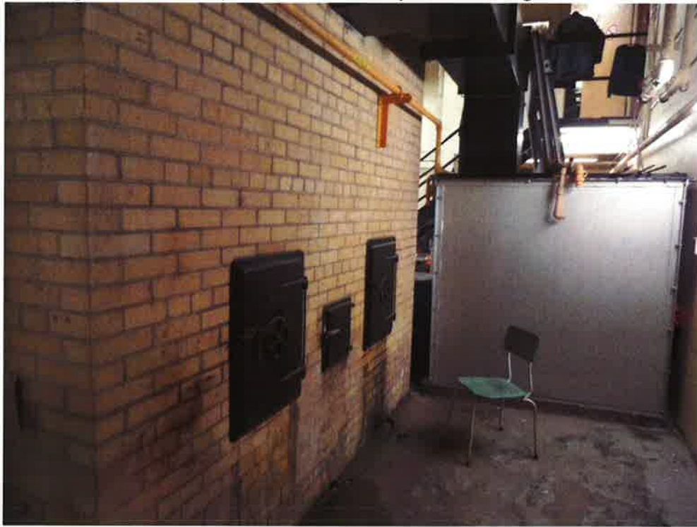
Photograph 9: Garbage incinerator, reported not to be in operation during the site reconnaissance.
