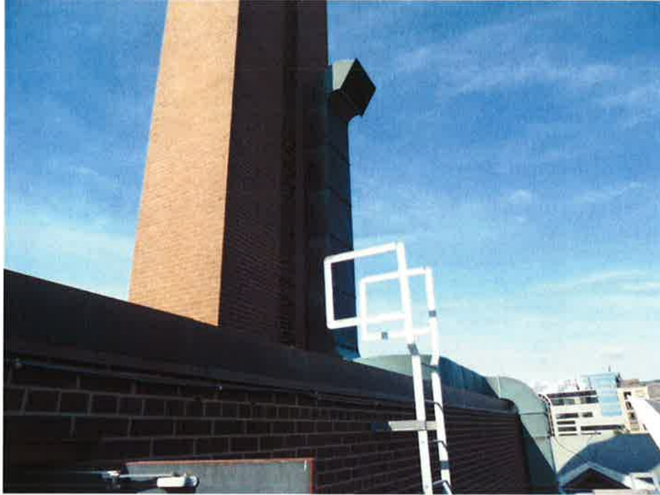
Photograph 3: Facing Southwest: The brick chimney that was used in the past for garbage incineration
