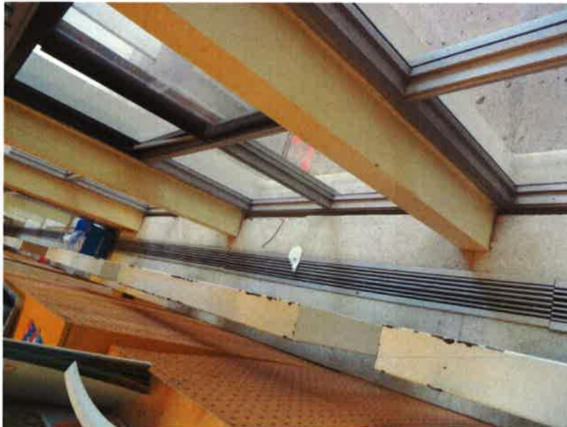
Photograph 10: Baseboard heating in one of the classrooms
