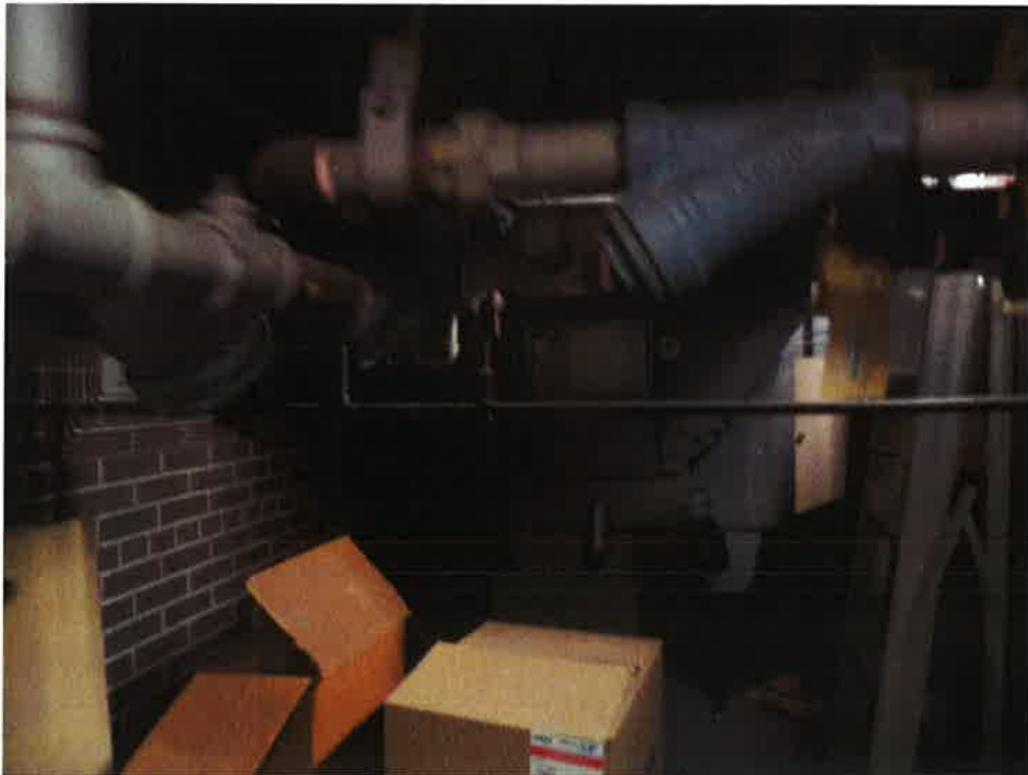
Photograph 4: View of the HVAC mechanical room
