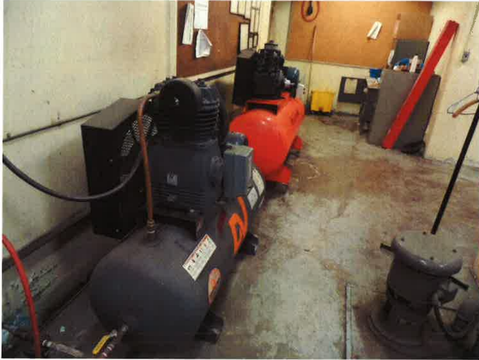
Photograph 7: Two compressors on the left and sump pump on the right. These units are located in the sub-basement.
